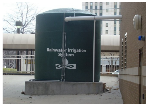
A cistern collects roof rainwater to irrigate the Employee Park.
