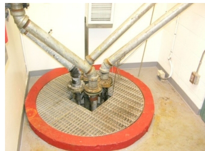
Groundwater is collected to supply the building's cooling system.
