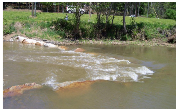
Carefully placed boulders direct flow to the stream's center, thus avoiding erosion impacts on stabilized banks.
